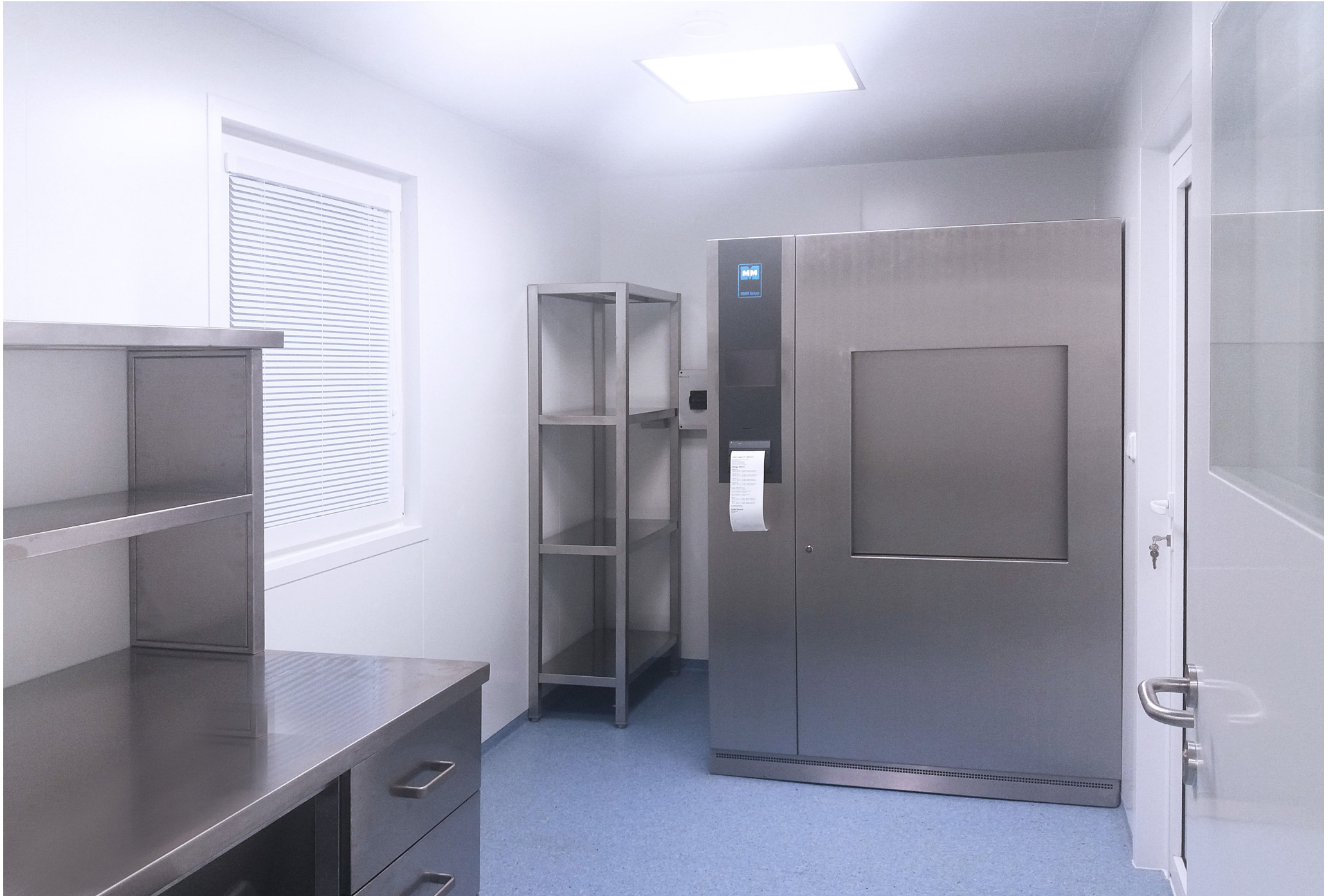
New Modern Boram General Hospital | VAMED Health Project CZ s.r.o. | Papua New Guinea | 2019
